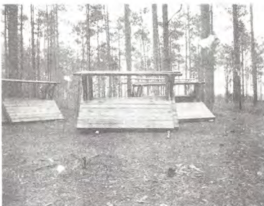
New Tent Platforms were constructed for one Troop site along with 5 new Patrol tables.
