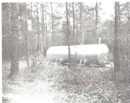
A new water system was installed which will be adequate to meet the needs of our total camp expansion program and the main camp. Picture is the new 5000 gallon water storing tank.
